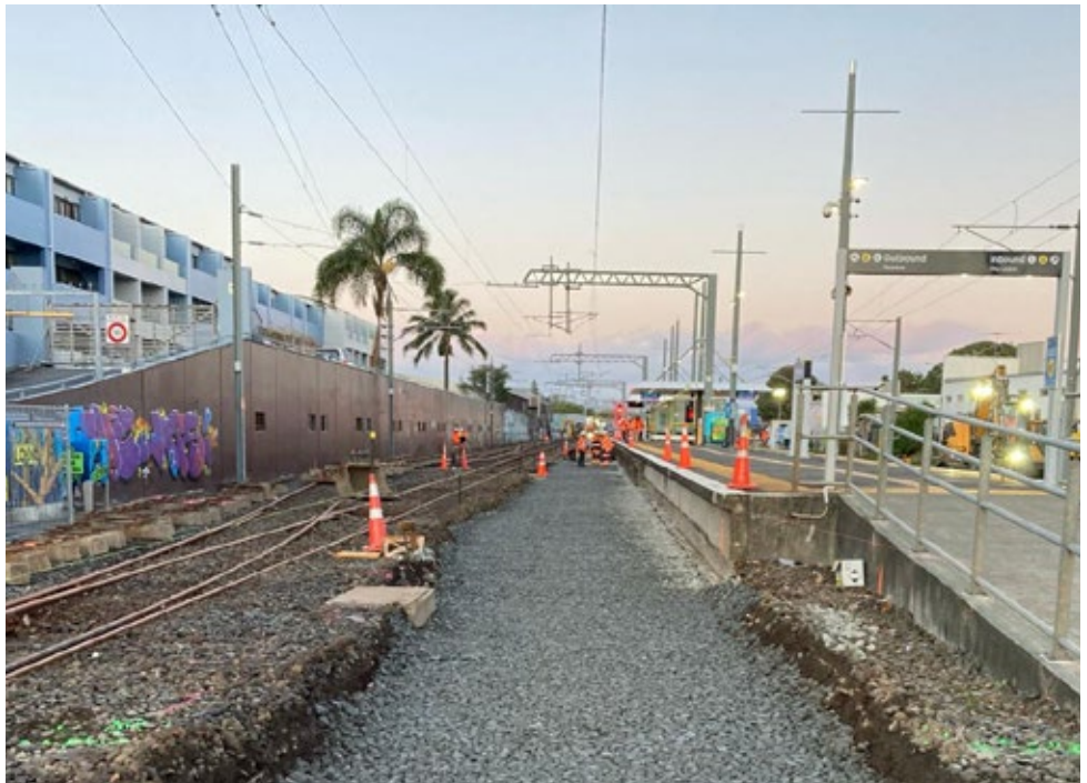
More than 12km of rail network foundations and 53km of drainage have been rebuilt so far on RNR
