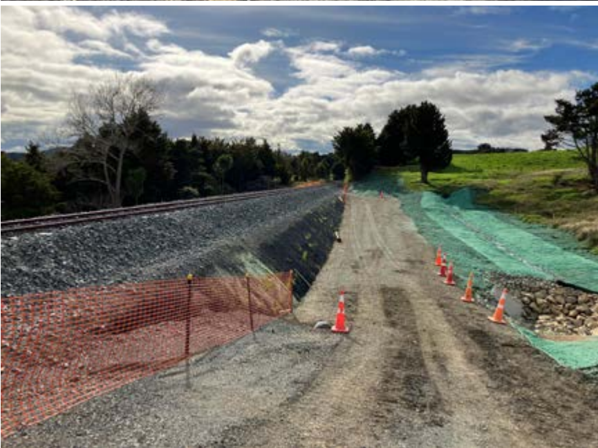
Progress repairing the major 185km damage site, south of Tauraroa. This is an example of Northland's slip prone geology, where a gentle hillside slumped under the rail line. It has required major excavation and drainage work beneath the rail embankment, which was rebuilt with sturdier materials.
