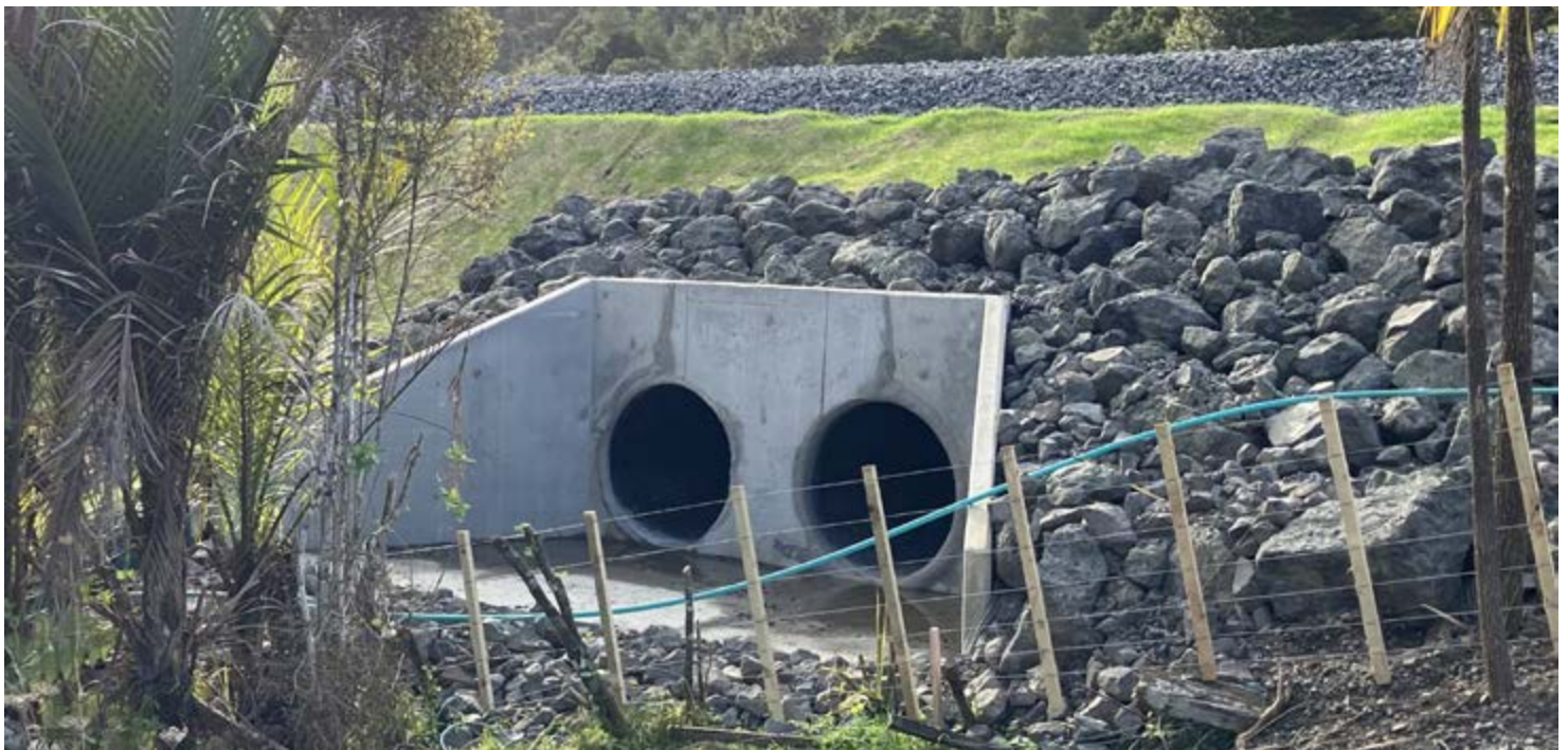
An example of drainage improvement near the 93km mark in the Ahuroa Valley. Installing larger culverts helps protect the line from being washed away in future weather events.
